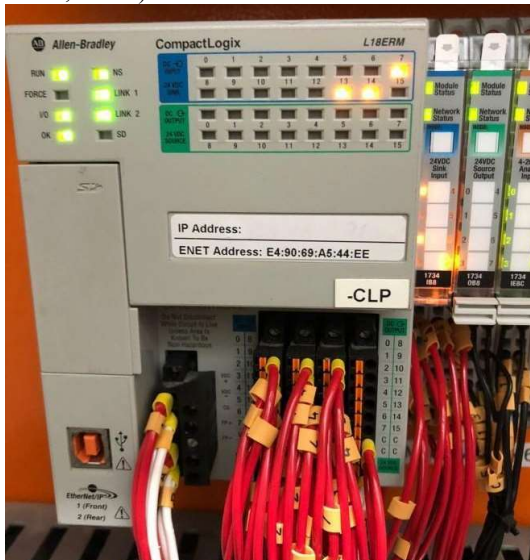
Figura02:CLP Allen-Bradley Rockwell.
